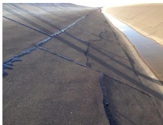
Uplift failure in cast-in-situ lining canal slope
