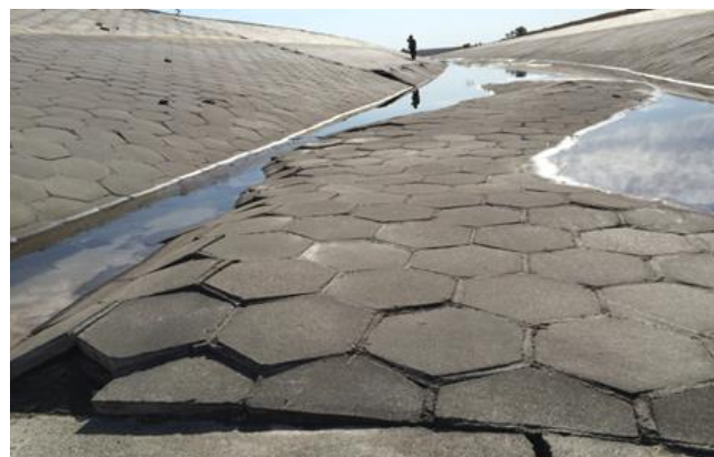
Uplift failure at the bottom of prefabricated lining canal
